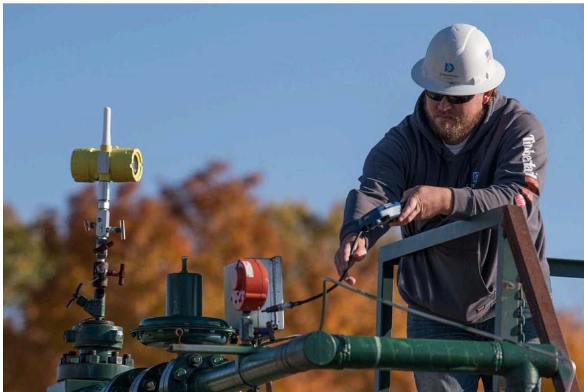
Diversified Energy says it reduced its methane intensity by 33% in 2023, compared to 2022, to 0.8 MT CO 2 e/MMcf and exceeded 75% of its 5-year goal for pneumatics conversions. (Source: Diversified Energy)
